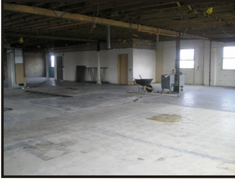
Beginning of renovations at LSS Faith Mission on 6th which were completed in October 2006.
